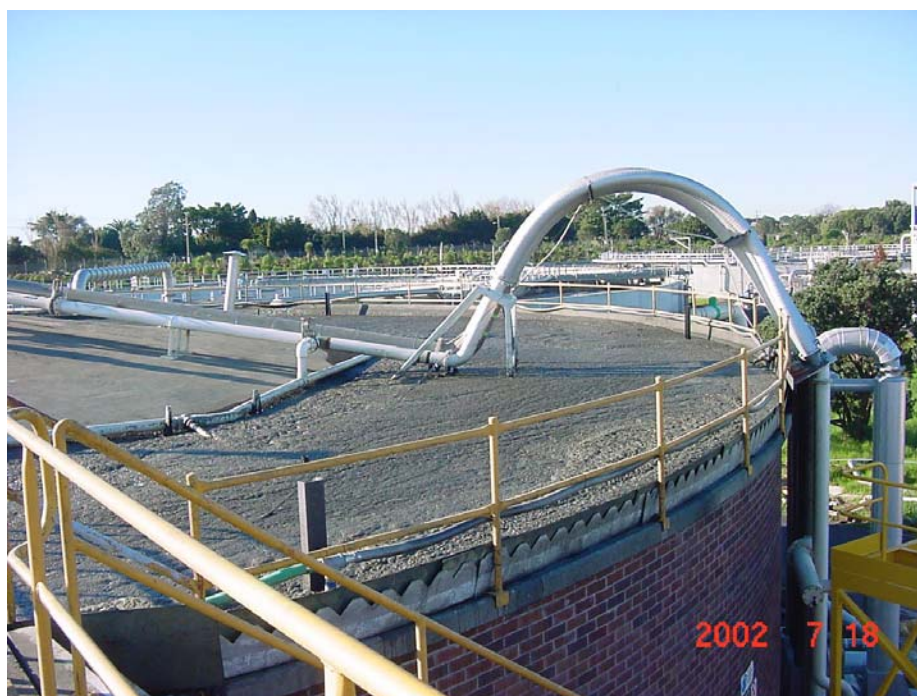
Photograph 1: Digester No. 6 Gas Collection Piping
