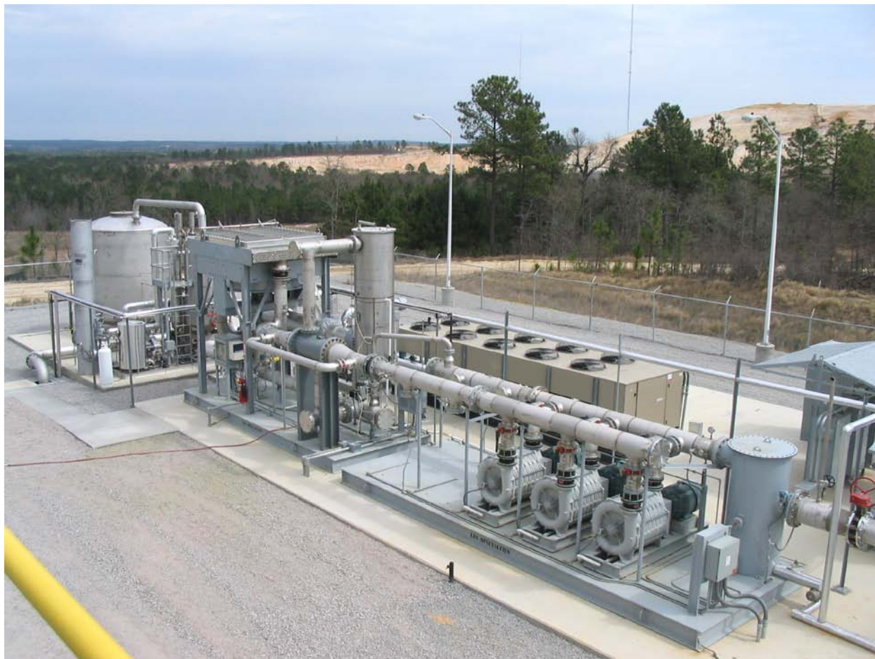
Richland, SC Landfill – 2500 SCFM
