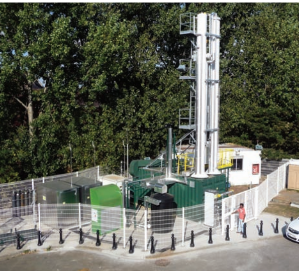
Water scrubbing in conjunction with pressure and temperature swing adsorption units removes CO 2 and H 2 S for the production of compressed biomethane for vehicle fuel. The Greenlane Biogas upgrading equipment (left) is installed at a facility in France.
